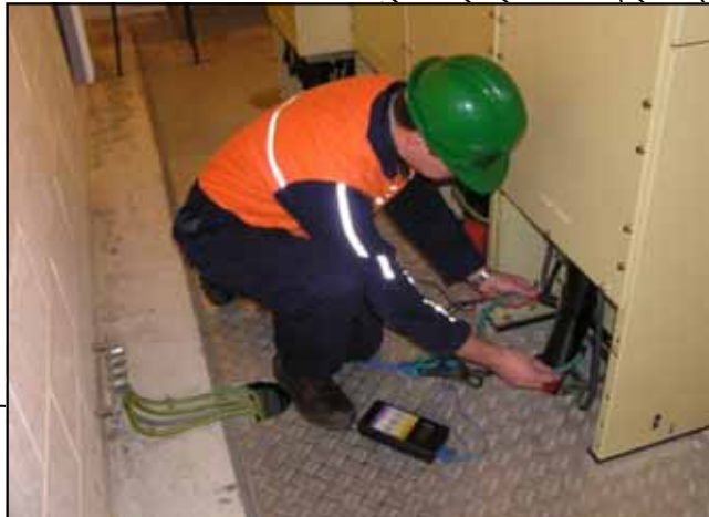
Measurement of 58 Hz current in 11 kV cable screen.
